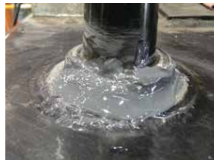
Sealed bushing leak
