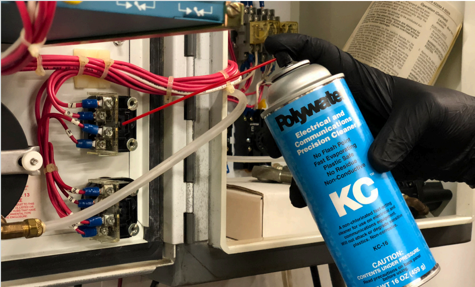
Cleaning an electrical contact
