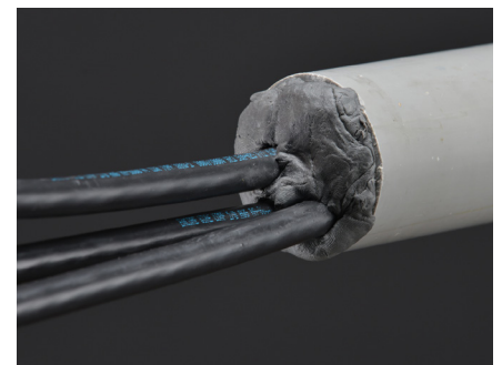
Damming prevents leaking
